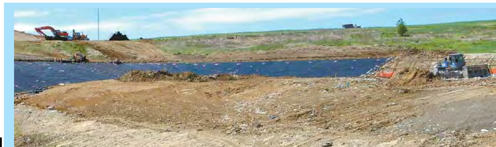
On the left side of this photo workers install an abutment liner on the side slope of the working face at the landfill while on the right side the compactor works on recently disposed of trash. The abutment liners are required under the most recent IDNR regulations.
